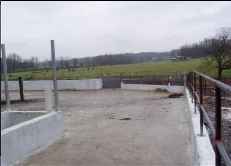
Heavy Use Area after stabilization. Cost share funds provided by the Districts 319 grant.
