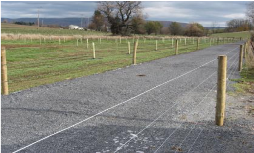
Pictured left shows a cattle access lane adjacent to new tree & shrub plantings which run along a Penn Creek tributary. The tree plantings and fence along the left side of the cattle access lane where cost shared through CREP. The cattle access lane and fence along the right side of the lane where cost shared with PVCA's National Fish & Wildlife Foundation grant funds.
